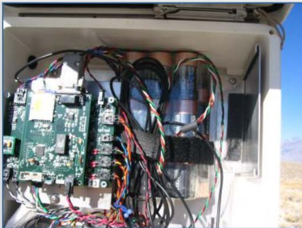
Figure 1: View of electronics and alkaline battery pack with enclosure mounted on tower
